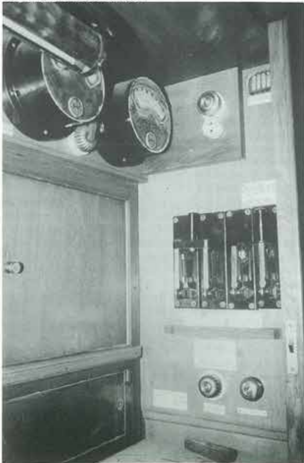
Switchgear to right of console.
